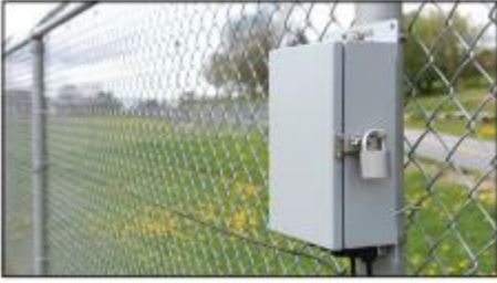
FlexZone processor on a fence
